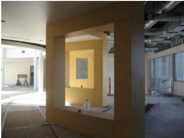
Display spaces under construction in the lobby will showcase beautiful geological specimens presented by generous donors.
