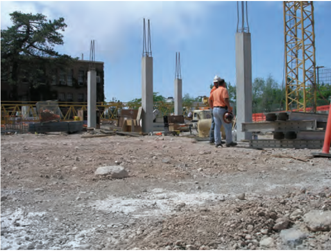
1. Sutton Building foundations are laid in the shadow of the 1927 Mines Building.
