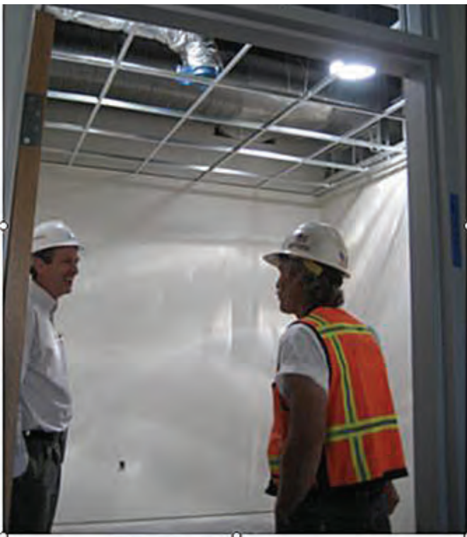
Architects and contractors helped make student conception of tubular skylights a reality.
