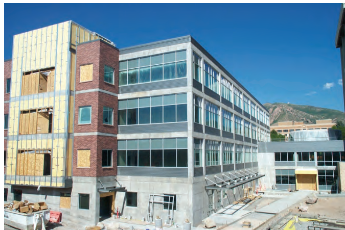
Developing construction finally gave us an idea how the Sutton building will fit into its campus environment.
