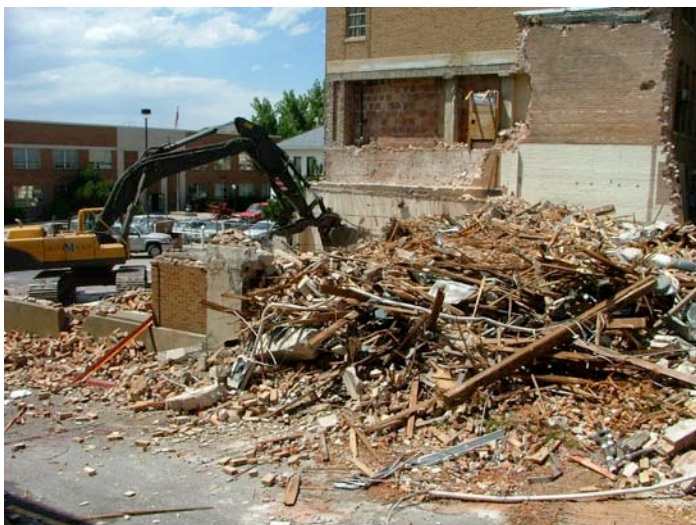
... and soon only a heap of rubble remained.
